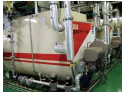
City gas boiler in the Karuizawa Plant
