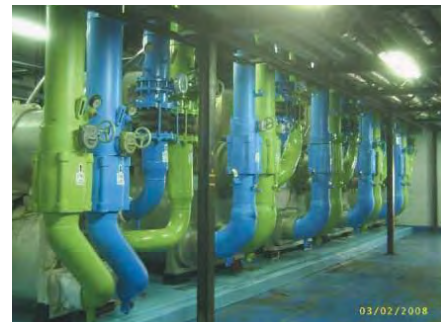
High-efficiency refrigerator installed in Bang Pa-in Plant (Thailand)
