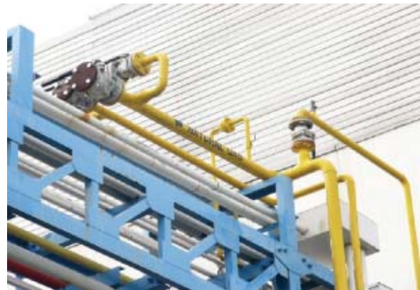
Natural gas supply line
