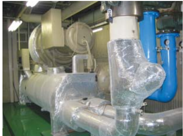
Newly introduced high-efficient refrigeration unit
