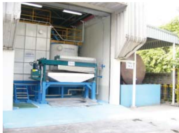
The Rojana Plant's new wastewater treatment facility
