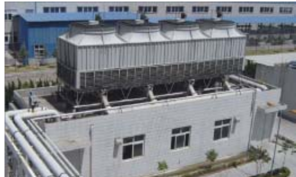
Shanghai Shunding Technologies' cooling tower
