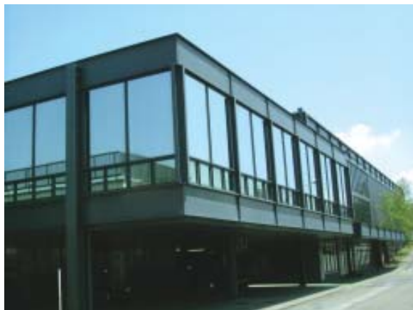
Shatter-resistant film on the windows of the Karuzawa Plant's cafeteria
