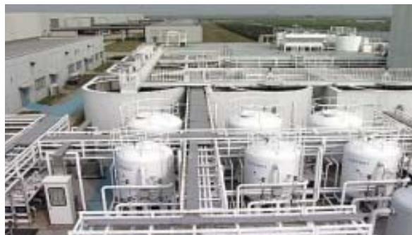
Wastewater treatment facility, Shanghai Plant (China)
