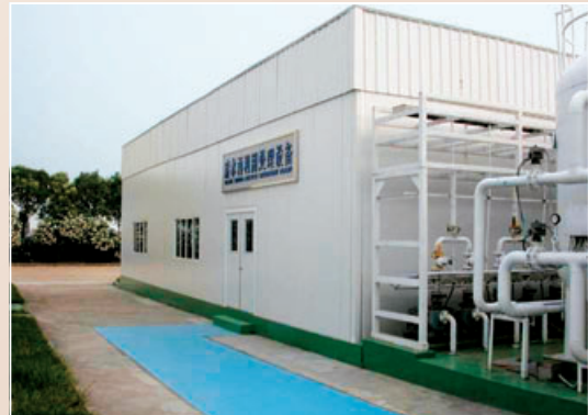
Wastewater recycling facilities (Shanghai Plant)
