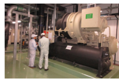
Centrifugal chiller installed in the Xicen Plant, China
