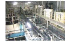
Fujisawa Plant's wastewater treatment facility
