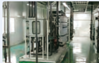
Effluent water treatment facility at our Shanghai Plant (began operation in Jan. 2009)
