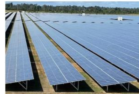
Solar power system already installed by SchneiTec
