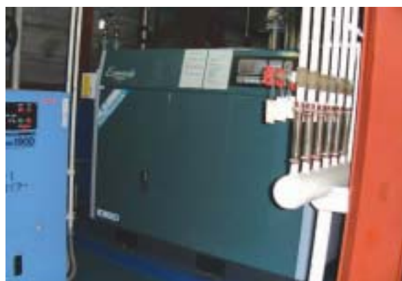
New compressors with inverters (Hamamatsu Manufacturing Unit)
