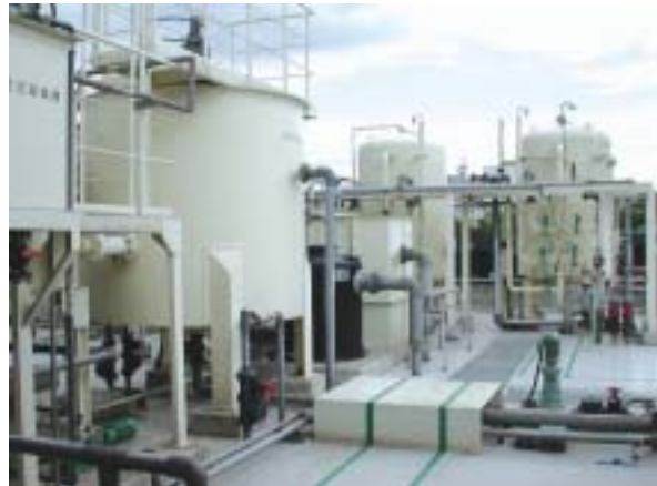
Comprehensive wastewater processing facility (Fujisawa Manufacturing Unit)
