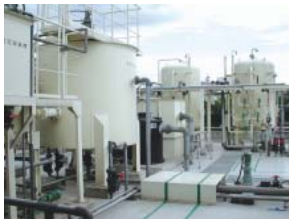
Comprehensive wastewater processing facility (Fujisawa Manufacturing Unit)
