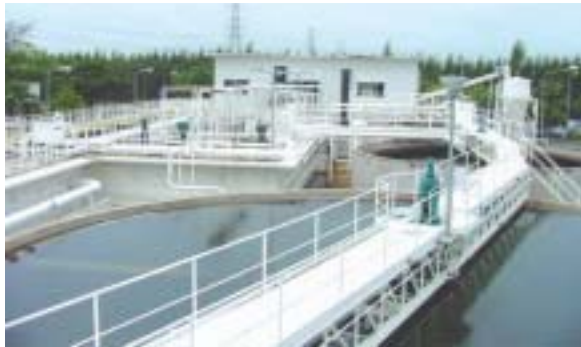
Wastewater treatment facility, Bang Pa-in Plant (Thailand)
