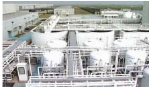
Wastewater treatment facility, Shanghai Factory (China)
