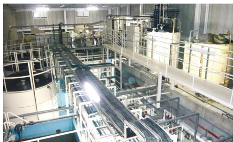
Fujisawa Plant's wastewater processing facility
