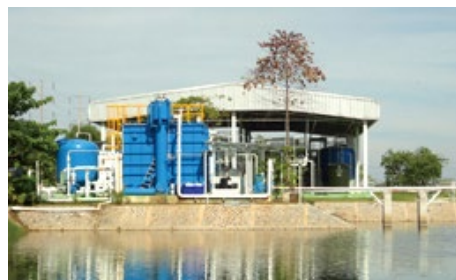
Bang Pa-in Plant's rainwater reservoir and rainwater reuse facility
